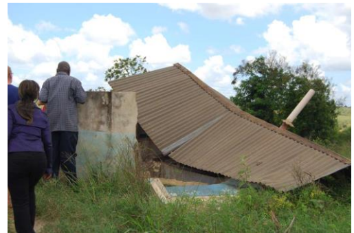
Collapsed toilet at Petanguo primary school
