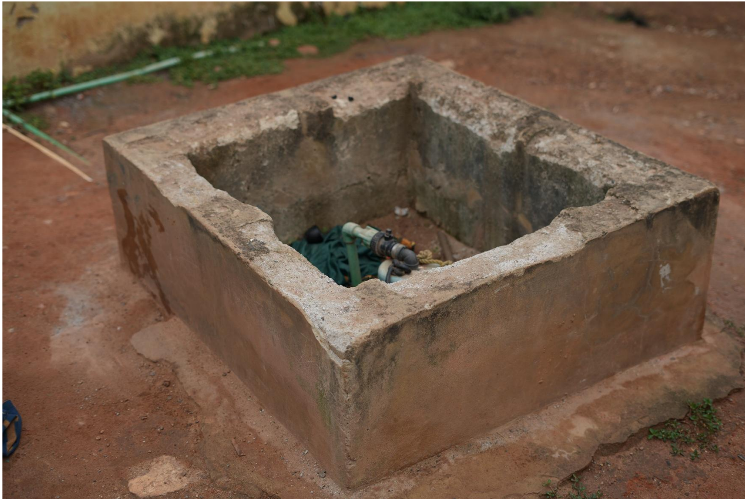
Figure 7: One of the non-working bore holes.
